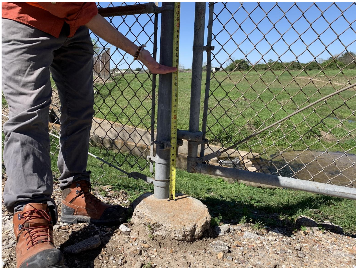
Figure 3: Reported HWM along fence near WWTP outlet
