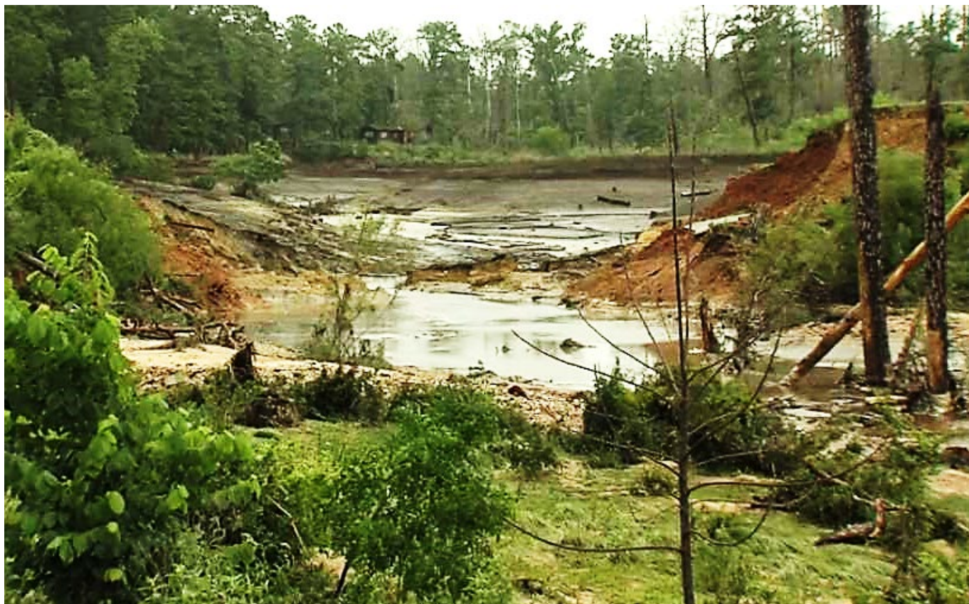
Failure of the Bastrop State Park Dam that was originally constructed in 1913 during the 2015 Memorial Day flood event. Source. Texas Parks and Wildlife.
