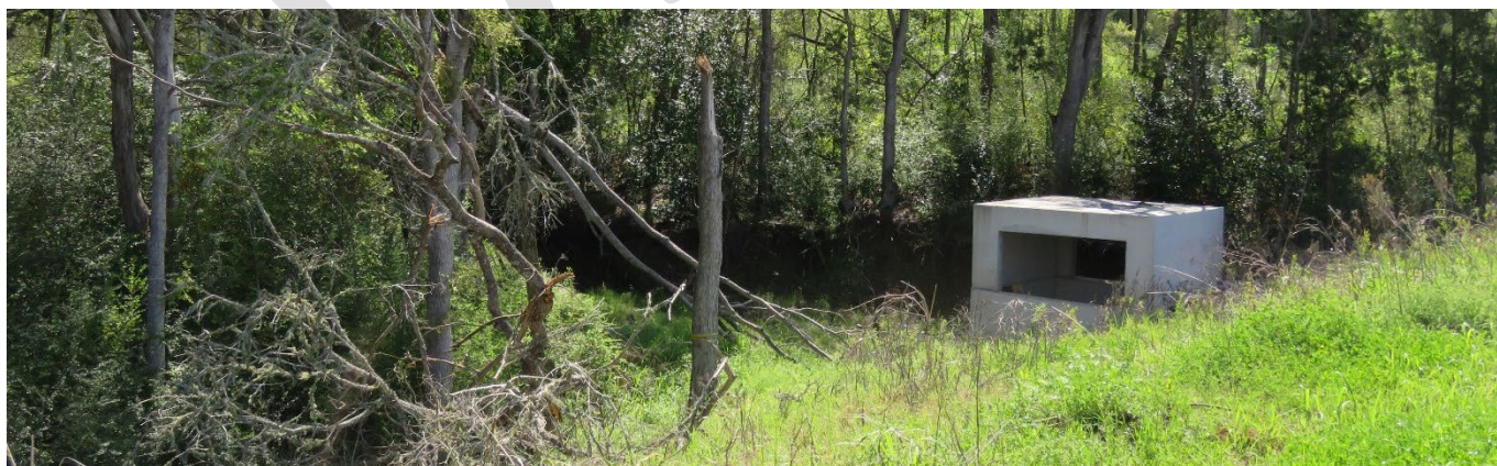
Drainage structures include such things as culverts to collect surface runoff and deliver it to underground stormwater conveyance systems.
