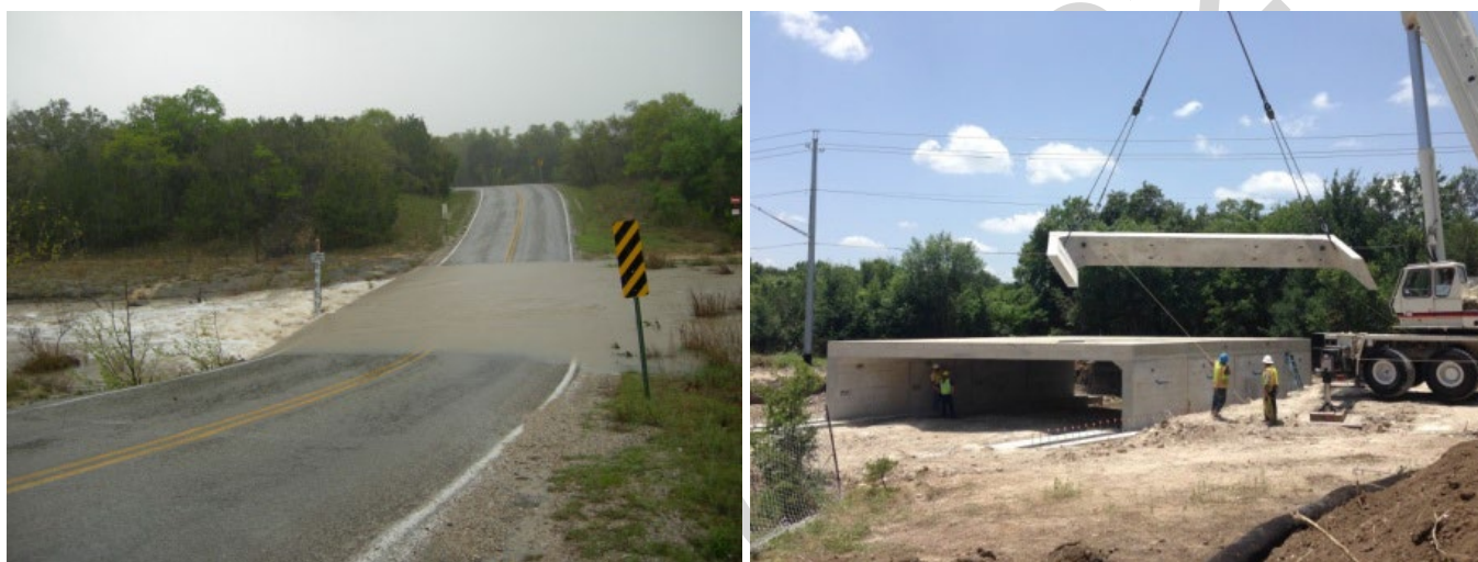
Example of Flooded Low Water Crossing at Bee Creek Road and Bee Creek in Travis County as well as an Example Low Water Crossing Upgrade with Precast Bridge Units, David Moore Drive, Austin
