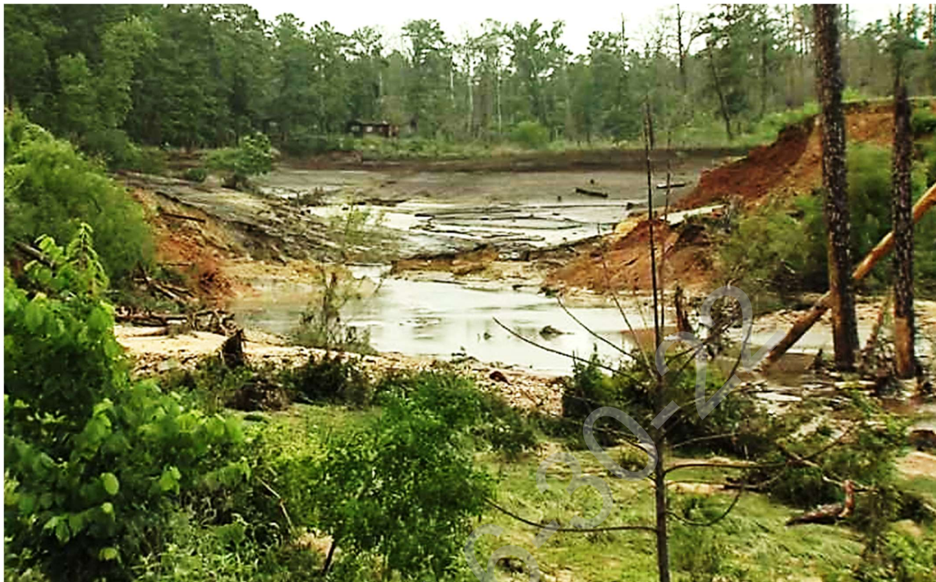
Failure of the Bastrop State Park Dam, which was originally constructed in 1913, during the 2015 Memorial Day flood event. Source. Texas Parks and Wildlife.
