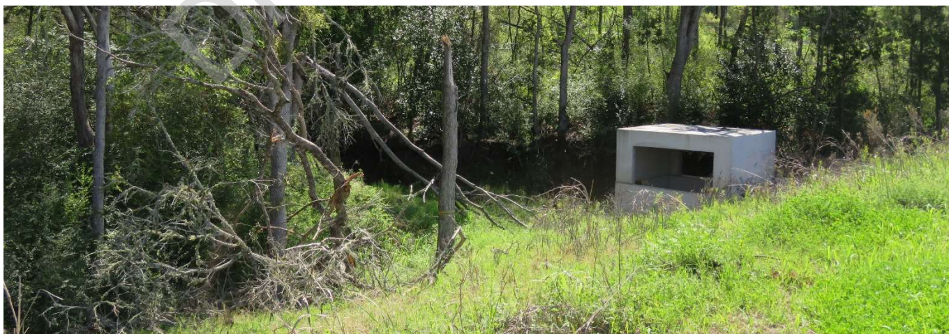
Drainage structures include such things as culverts to collect surface runoff and deliver it to underground stormwater conveyance systems.
