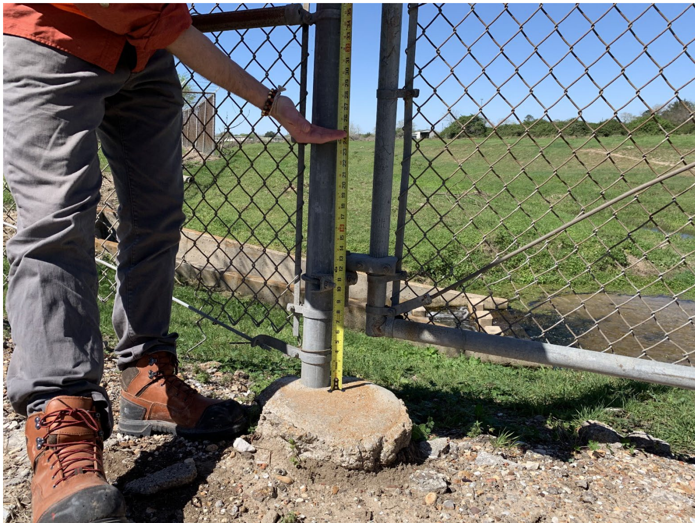
Figure 3: Reported HWM along fence near WWTP outlet
